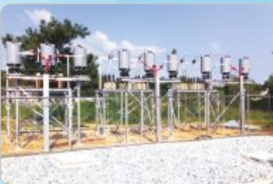
HT Harmonic Filter Capacitor Bank
