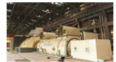
CPI Lanzhou New District Co-generation of Heat and Power Project
